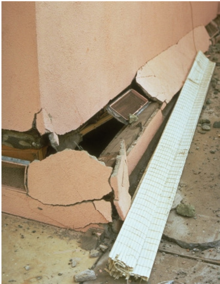
Figure 2-5 Typical earthquake damage to a cripple-wall house (from ATC, 2002).
