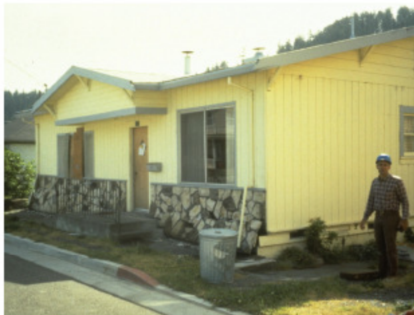
Figure 2-13 Damage to a basement-type house where the sill plate slid on the top of the foundation wall (from ATC, 2002).
