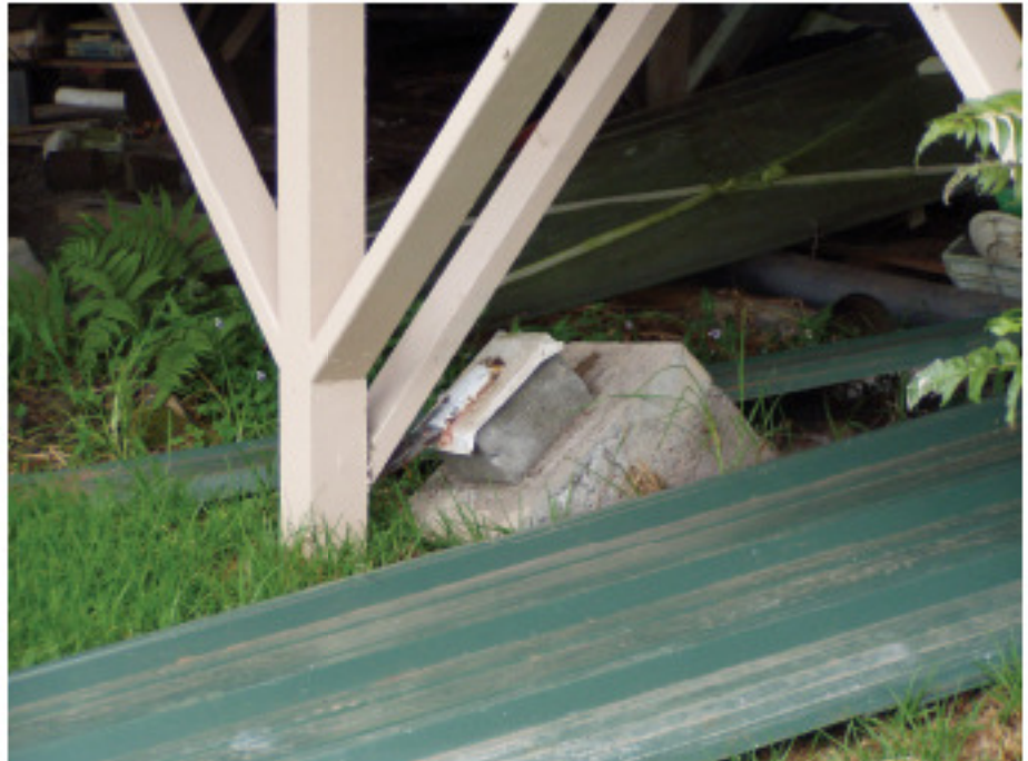
Figure 2-17 Earthquake-damaged perimeter post-and-pier foundation. The diagonally-braced post has overturned the shallow-founded concrete pier footing (from ATC, 2002).
