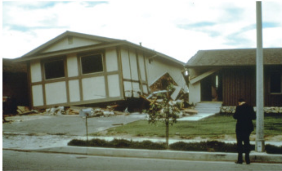
Figure 2-19 Split-level house with damage and collapse at the garage-level walls at two-story portion (from ATC, 2002).
