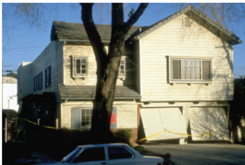
Figure 2-10 Damage and racking displacement to the right in the first floor walls of a two-story slab-on-grade house (from ATC, 2002).
