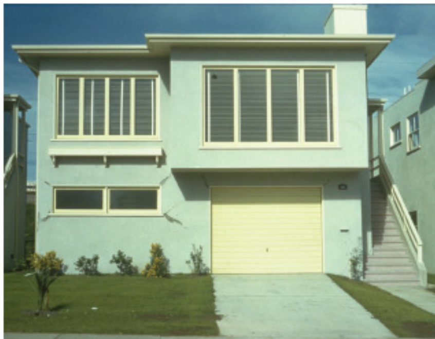
Figure 2-9 Cracking damage at the window to stucco first-floor walls of a two-story slab-on-grade house (from ATC, 2002).
